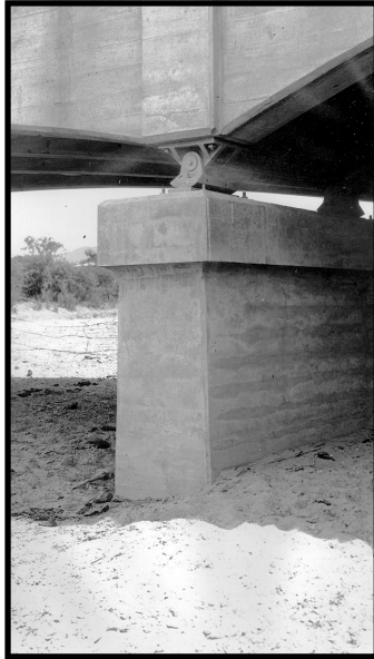
Figure 12. The eastern-most pier on the Continental Bridge at the Santa Cruz River as seen from the north side of the bridge. Elevation: 2818 feet.
